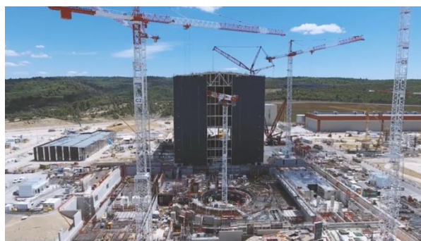
© ITER Organization, http://www.iter.org/
